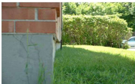
Building damage: Note displaced bricks and inward deflection of foundation. U.S. Army Corps of Engineers Photo. https://geology.com/articles/expansive-soil.shtml
