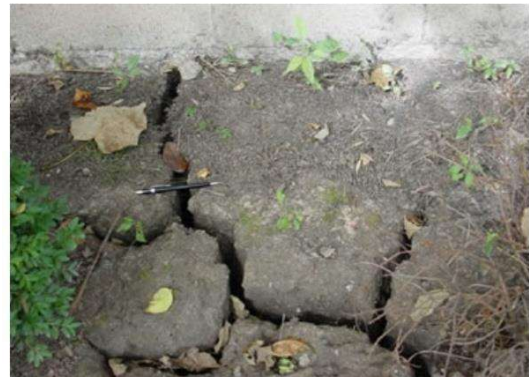
Cracks in expansive soil: Desiccation cracks in soil caused by drying. U.S. Army Corps of Engineers Photo. https://geology.com/articles/expansive-soil.shtml
